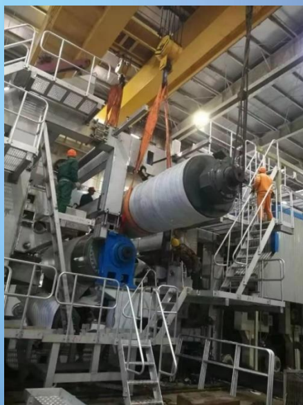
Four Rolls Three Presses 四辊三压 改造
